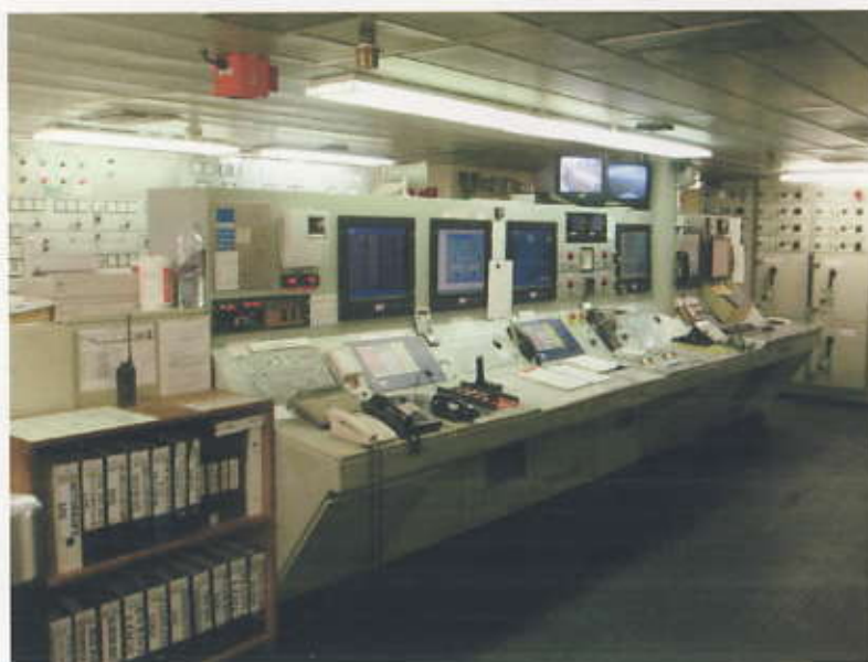
ARTEMIS Engine Control Room
